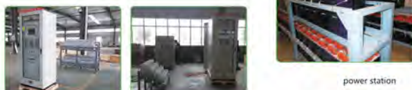
110V System & 48V System
